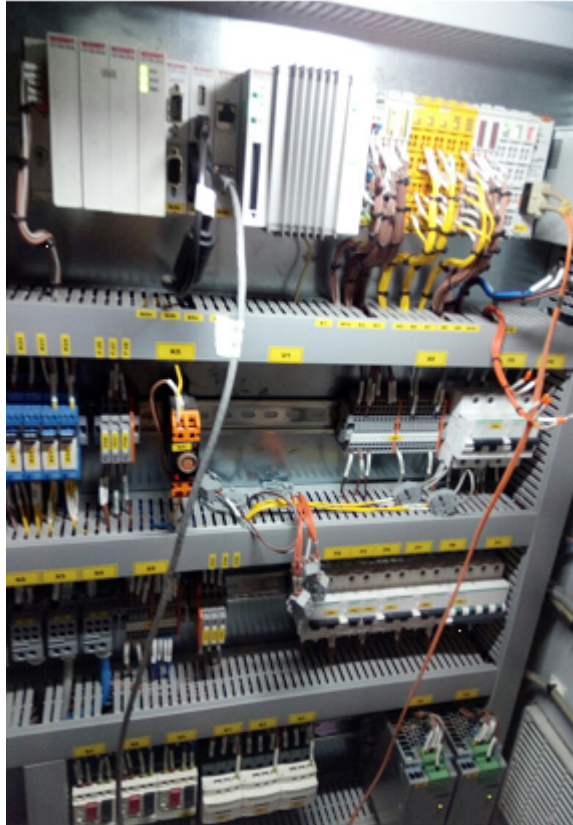
Figure 4.6: BECKHOFF CX1020 Controller panel
