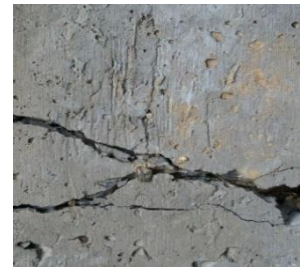
(i) Concrete wall image 9 with cracks, dents, texture, and stain marks
