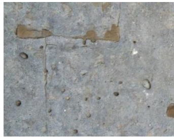
(b) Concrete wall image 2 with crack, dents, and noises
