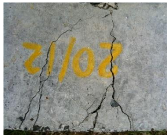
(e) Concrete object image 5 with cracks, noises, texture, and coloured numerals
