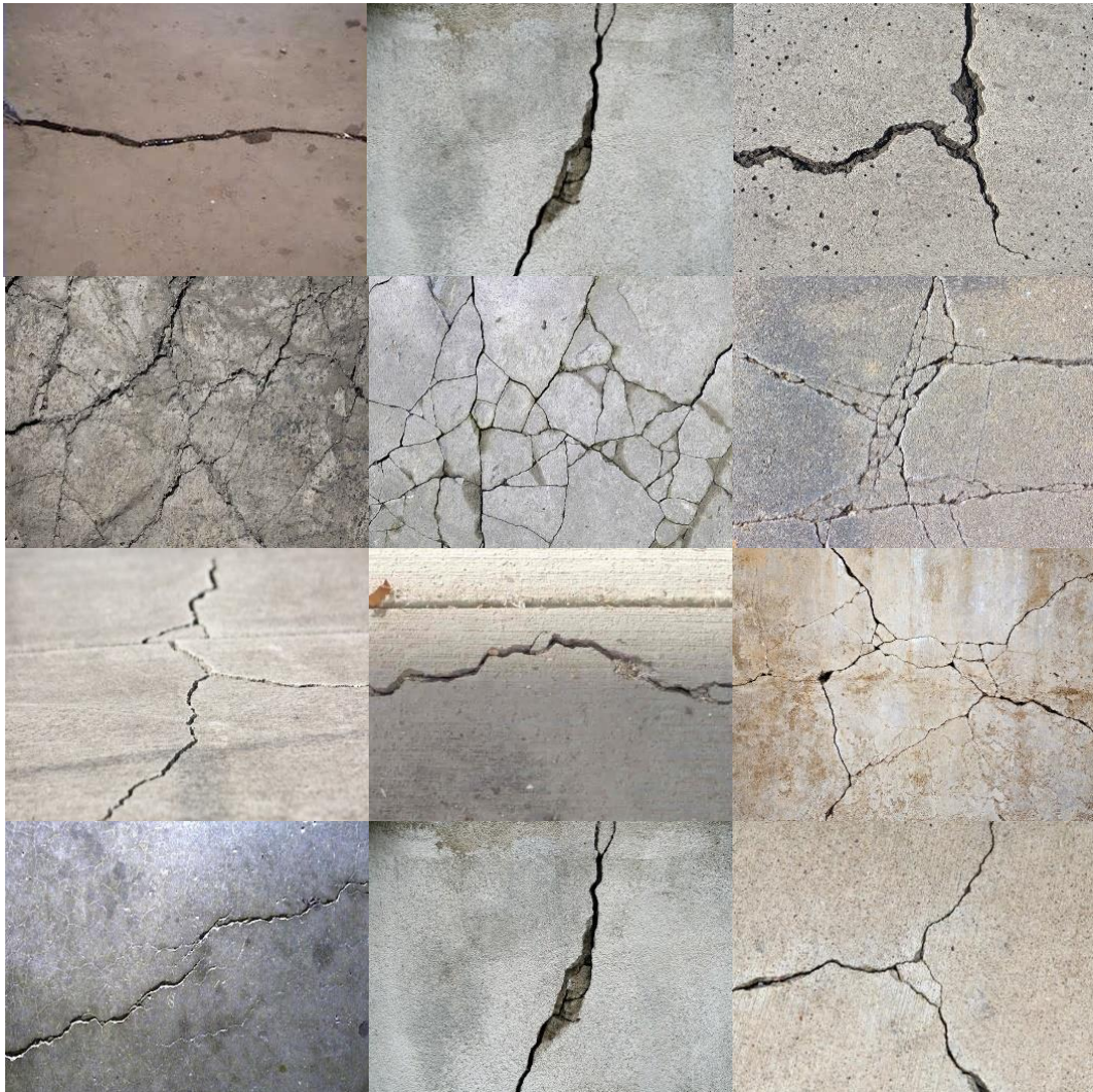
Figure 1. Sample concrete crack images.
