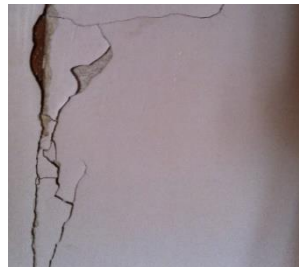
(h) Concrete wall image 8 with cracks, texture, shadow and stain marks
