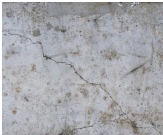
(d) Concrete sample image 4 with crack, noises, blemishes and texture
