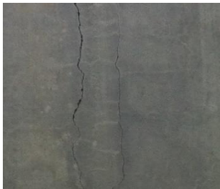
(g) Concrete object image 7 with cracks, and texture
