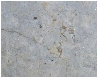
(a) Concrete wall image 1 with crack, dents and noises
