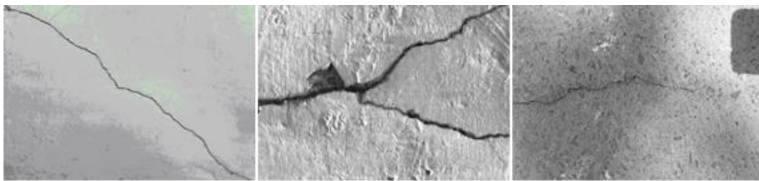
Figure 52. Testing images of surfaces with crack.
