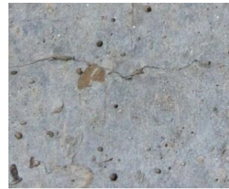
(c) Concrete wall image 3 with crack, dents, and noises
