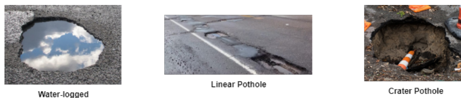
Figure 3.3: Varieties of Potholes
