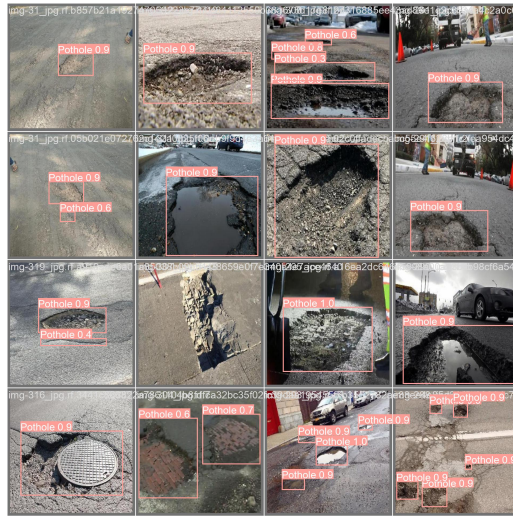
Figure 4.6: Predicted Potholes for YOLOv8
