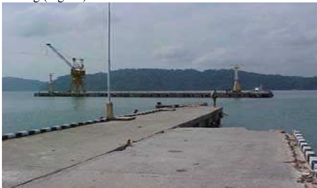
Fig. 7 Collapse of the 80 m segment of approach in Great Nicobar Island jetty at Campbell Bay.
