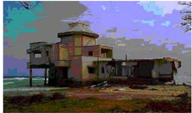
Fig. 5. RC frame building (MES Inspection Bungalow) now stands in waters at the Military Residential Colony south of Malacca on the east coast of Car Nicobar Island.
