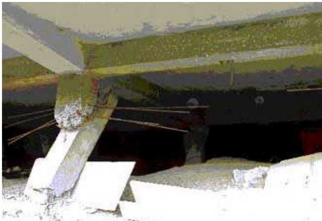
Fig. 6. Collapse of a three-storey reinforced concrete frame building at Port Blair
