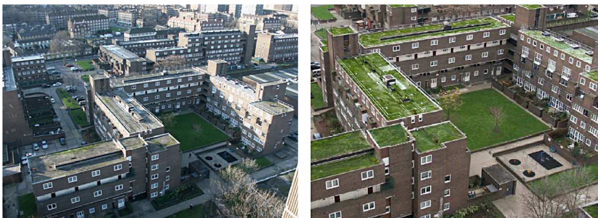
Fig.3 Original flat roofs at Ethelred Estate and green sedum roofs after refurbishment.
