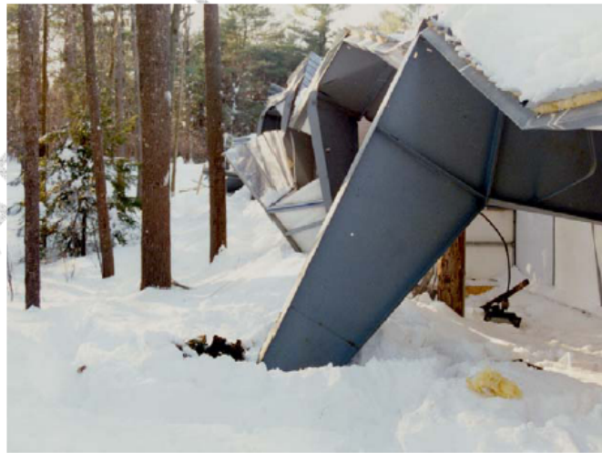
Figure 1.5: Failed bents looking in direction of progressive collapse
