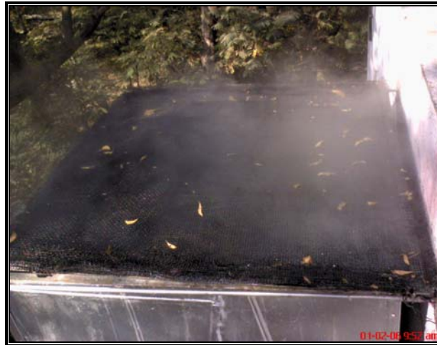
Fig. 3.3.1.5.1: Water Vapor coming out from the Duct (D1)
