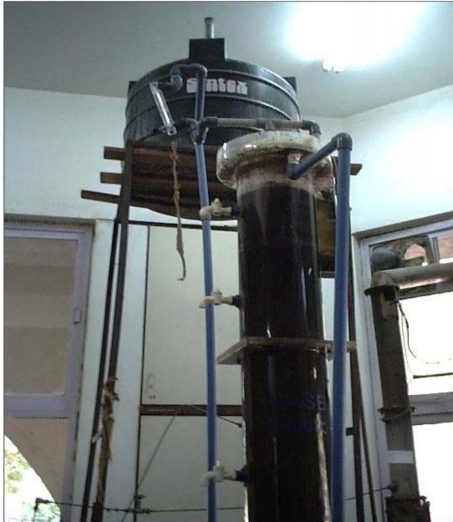
Figure: 4.1.1. Influent collection system
