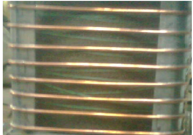
Fig. 1 View of Evaporator
