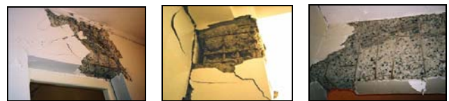
Fig. 17: Poor Quality of Materials
