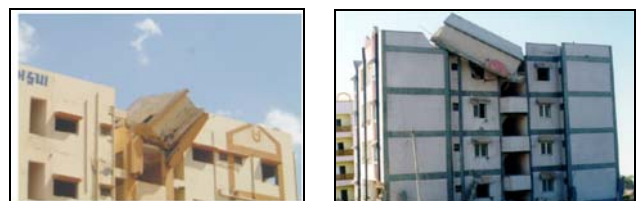
Fig. 10 Water Tank at roof causing structural damage
