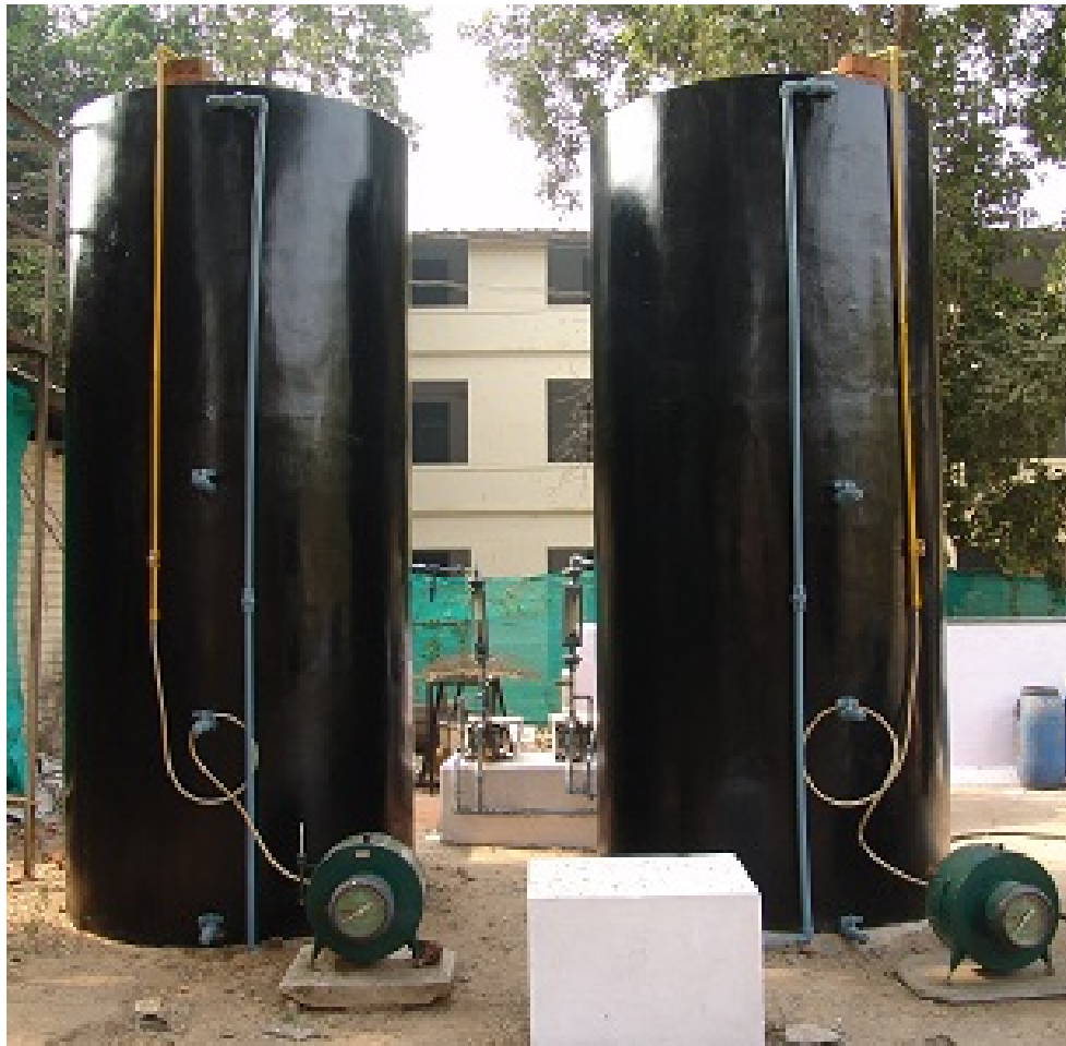
Figure 3.3: Pilot Anaerobic Filters
