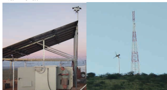
Figure-1: Wind/Solar installation in Namibia Left: Solar Array, Battery & Power Controller Right: Wind Turbine
