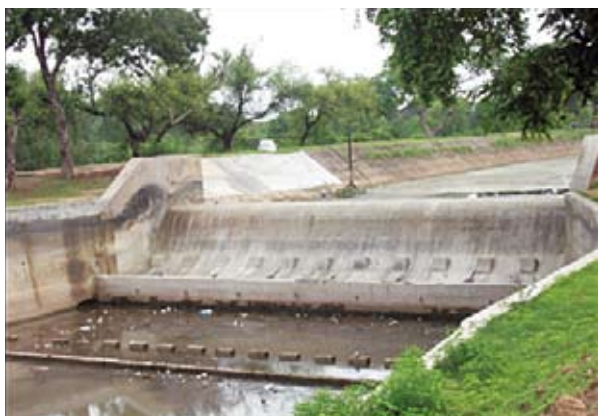
Fig 2 Fall at chainage 33,800 m
