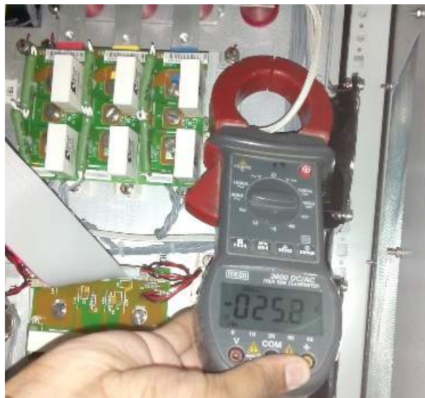
Figure 10.10: Load Current Measured using ACCT
