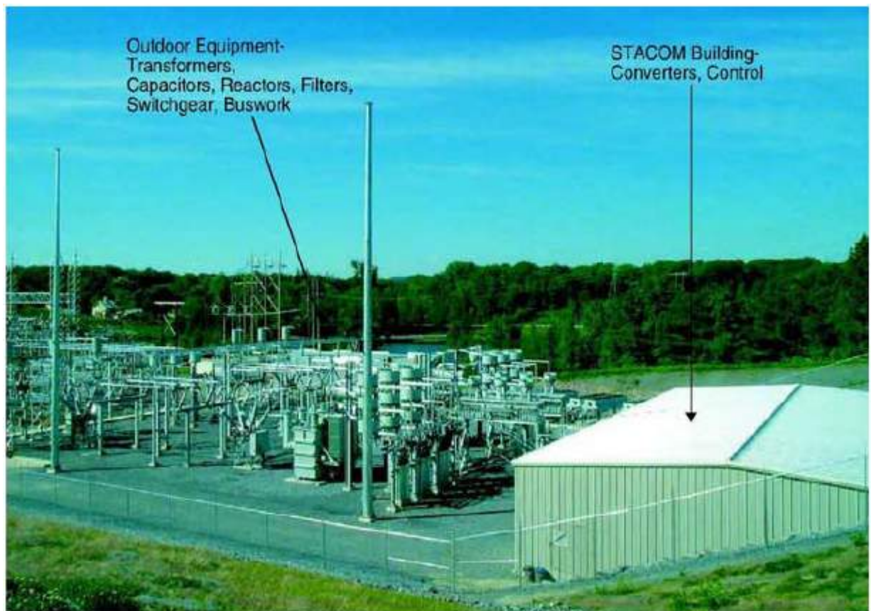
Figure 3.12: Essex project- external view +133/-41 MVA, 115 kV STATCOM system
