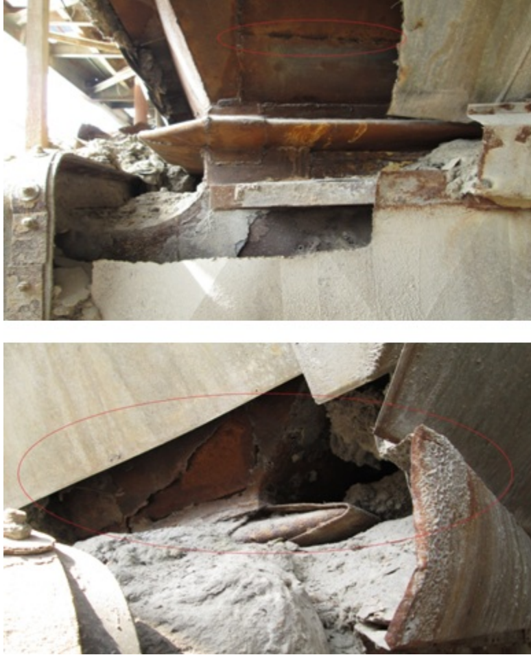
Figure 4.8: Damage of APH
