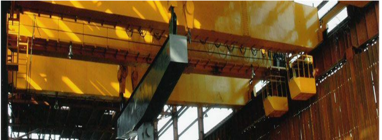
Fig 3 EOT(ELECTRIC OVERHEAD TRAVEL) CRANE
