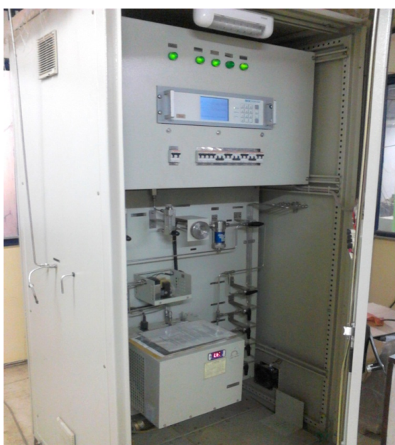
Figure 3.3: Photograph of a CO-CO 2 Analyzer
