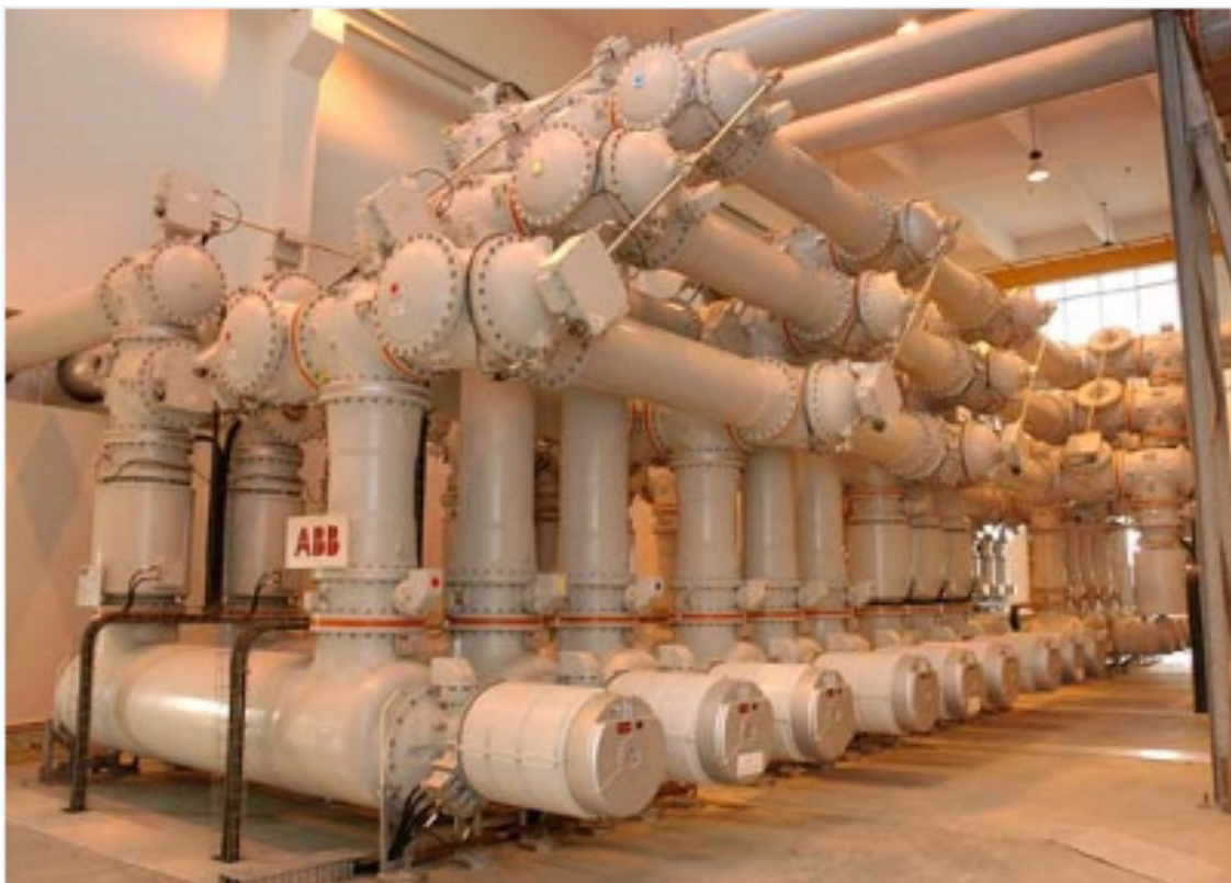
Figure 1.1: Gas Insulated Substation [13]
