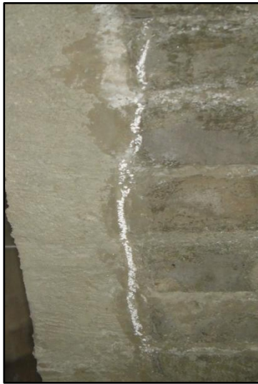
(A) Separation of Mortar Bond at Column Face
