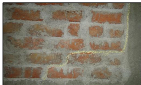
(B) Stepped type of failure
