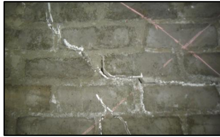
(B) Stepped Failure
