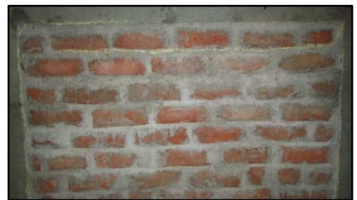
(C) Failure of horizontal mortar joint.
