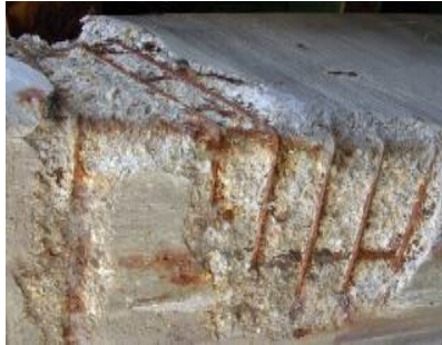
Figure 5 Acid attack on concrete
