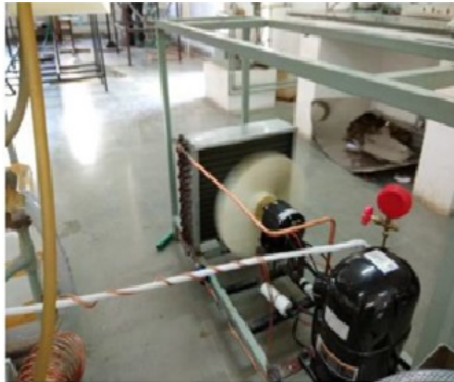
Figure 3.4: Refrigeration System showing compressor, coming from heat exchanger. capillary tube, condenser and condenser fan.
